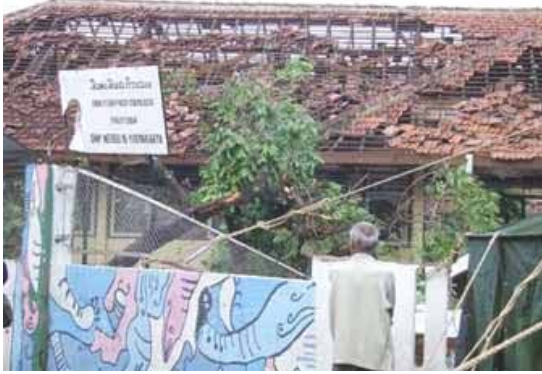
Figure 14. Loose tile roof, need formal code
