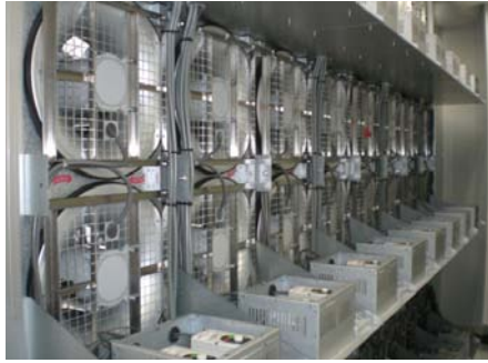
(a) Multi-fan room
